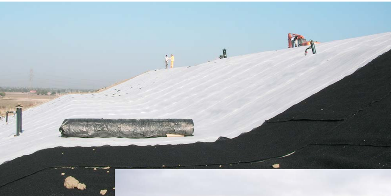
Final capping of Gello ITALY (Pisa), 2011-2013 MacDrain W 1081 drainage geocomposite used as soil gas drainage and as rainfall water drainage in the final capping lining.
